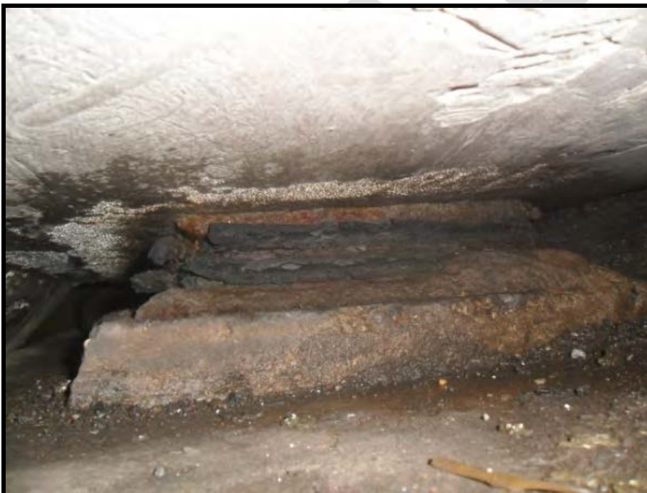
(Failure of elastomeric layers, loss of movement ability)
