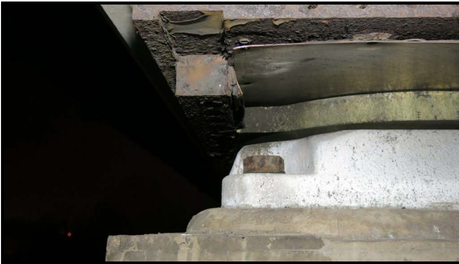
(Corrosion causing deformation of sliding surfaces, restrict movement)
