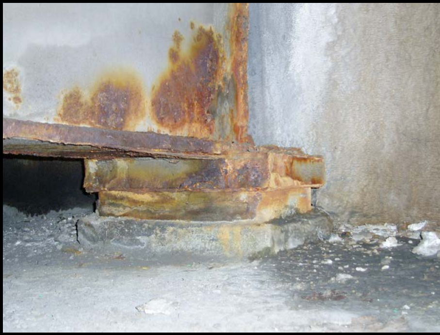
(Corrosion, loss of section and reduction in strength)
