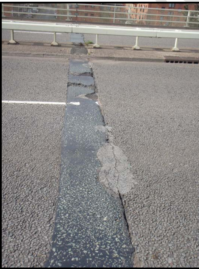
(loss of material and cracking, water ingress to structure and bearings below)
